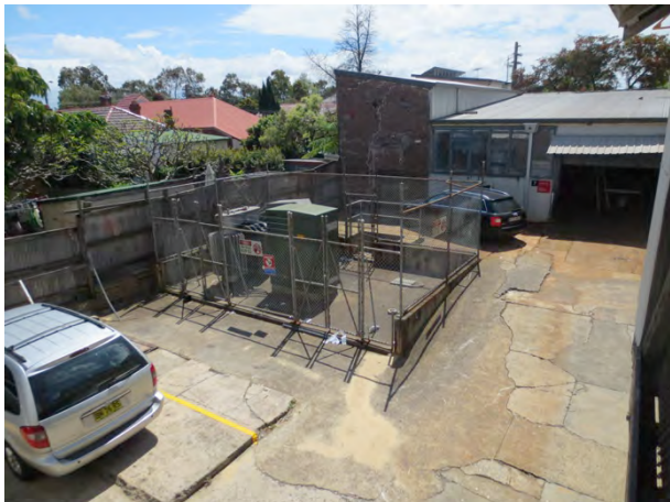
Substation behind Building 7.
